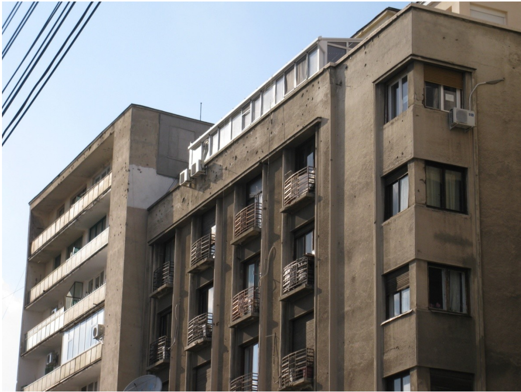
The bullets are still visible on many buildings surrounding the Revolution Square, like on the one captured here (Bucharest, March 2010).
