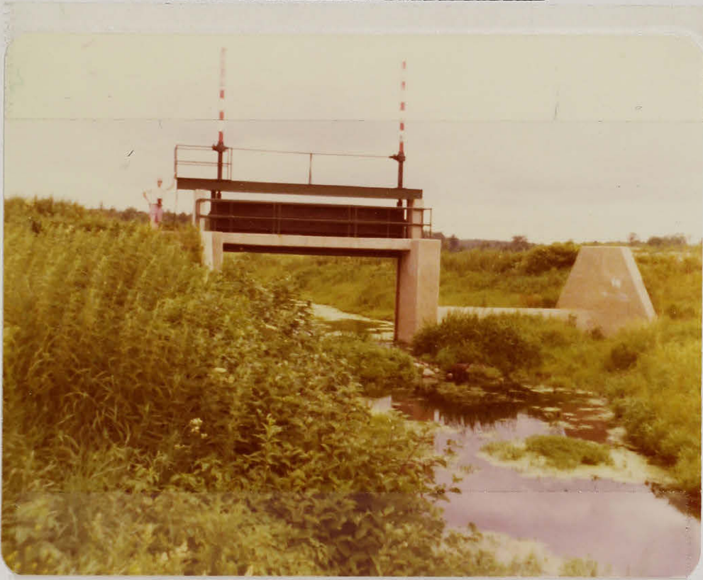
PHOTO 1. Water table control dam on Cranberry Creek
