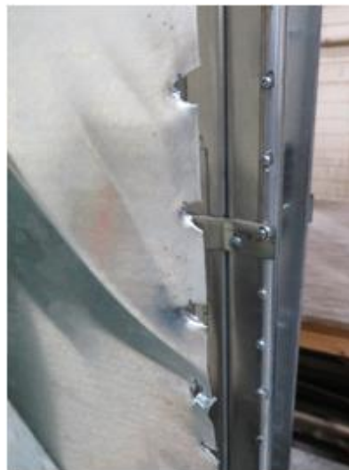
Figure 2.17 Screw tear-out failure
