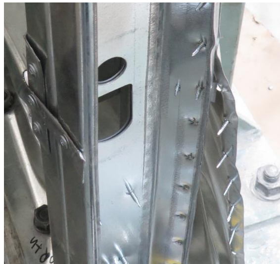
Figure 2.15 Sheathing screw pull-out failure
