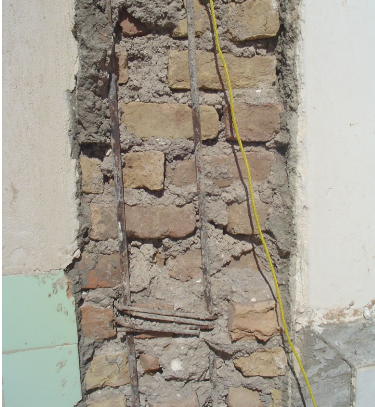
Figure 3.22. Reinforced concrete column with poor concrete mix, inadequate steel bars, and poor execution. Photo: HFIR archive
