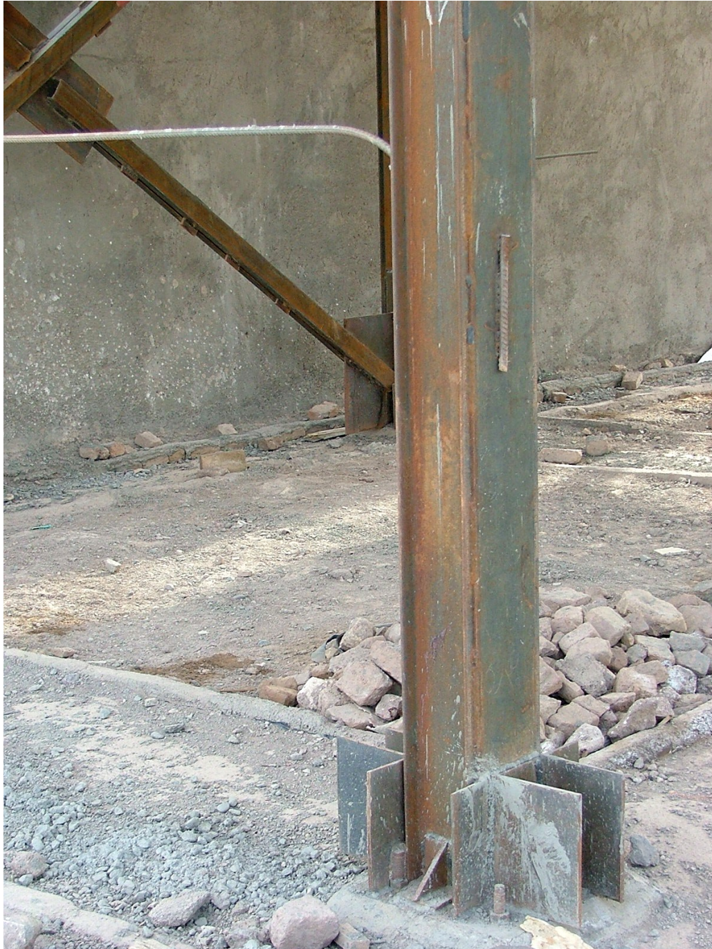
Figure E.13. An example of a column, oversized and overdone by the builder for the sake of a stronger structure
