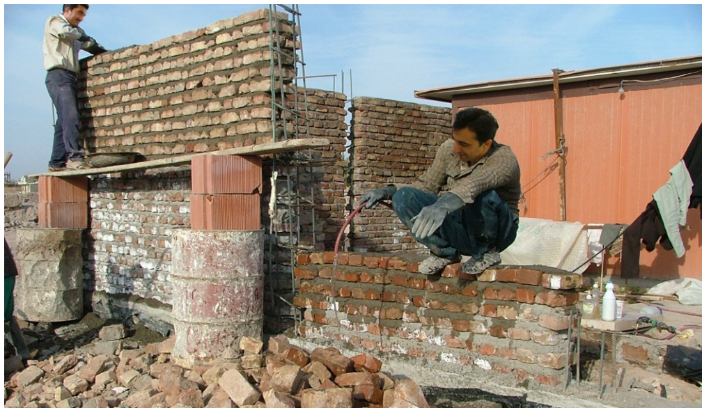
Figure 3.45. Sprinkling water onto the pile of bricks instead of soaking them
