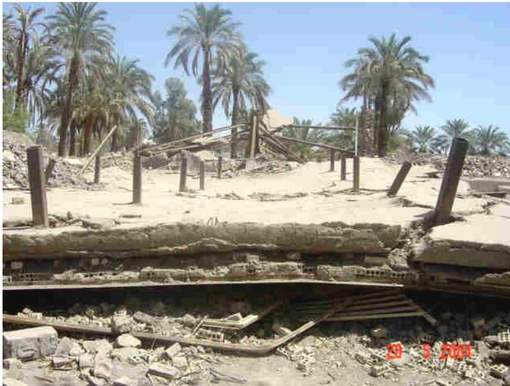
Figure 3.8. A flat roof collapsed due to its heavy weight and poor shear connection. Photo: HFIR archive
