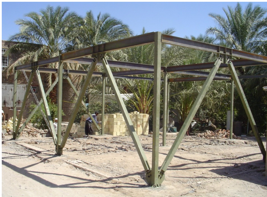
Figure C.1. After 15 months, not many houses were completely reconstructed. Photo: HFIR archive
