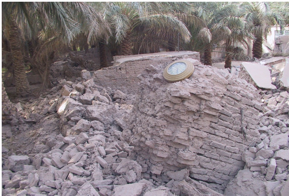
Figure 3.13. Poor quality of adobe, crushed into small pieces. Photo: HFIR archive
