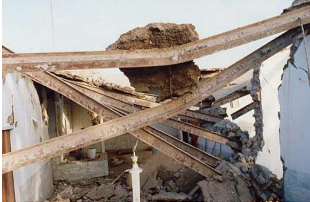
Figure 3.9. Roofing system incompatible with the load bearing elements (walls). Photo: ISEO 2004
