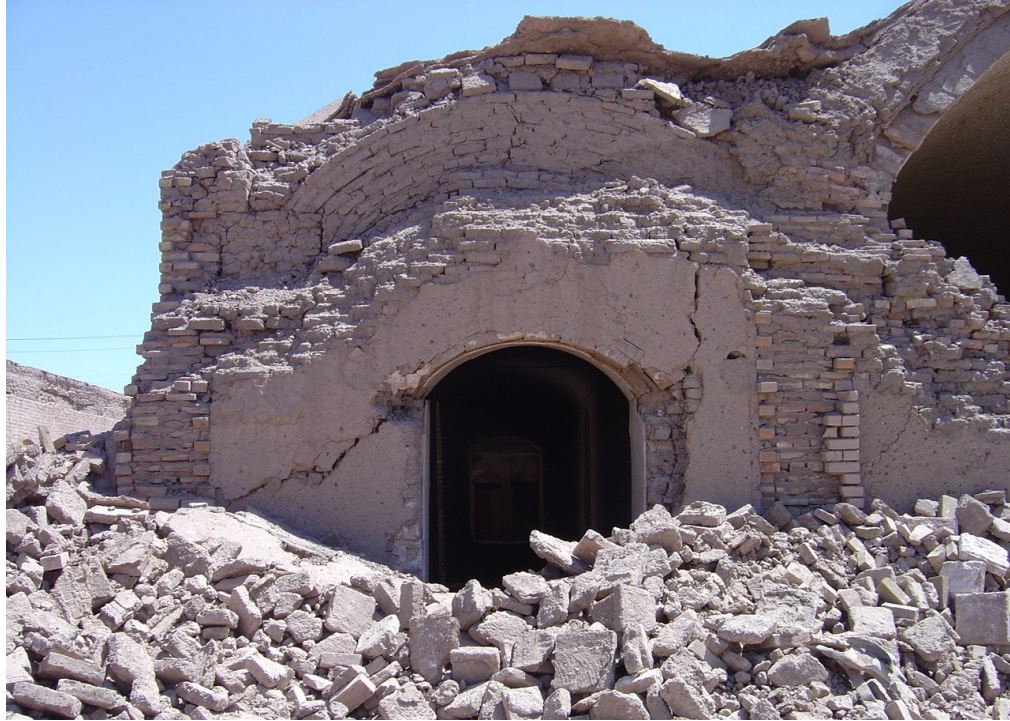
Figure 3.7. An earthen roof collapsed due to its heavy weight. Photo: HFIR archive
