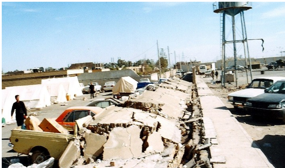
Figure 3.3. Even thick walls are destroyed when there is no pilaster along a long wall. Photo: HFIR archive
