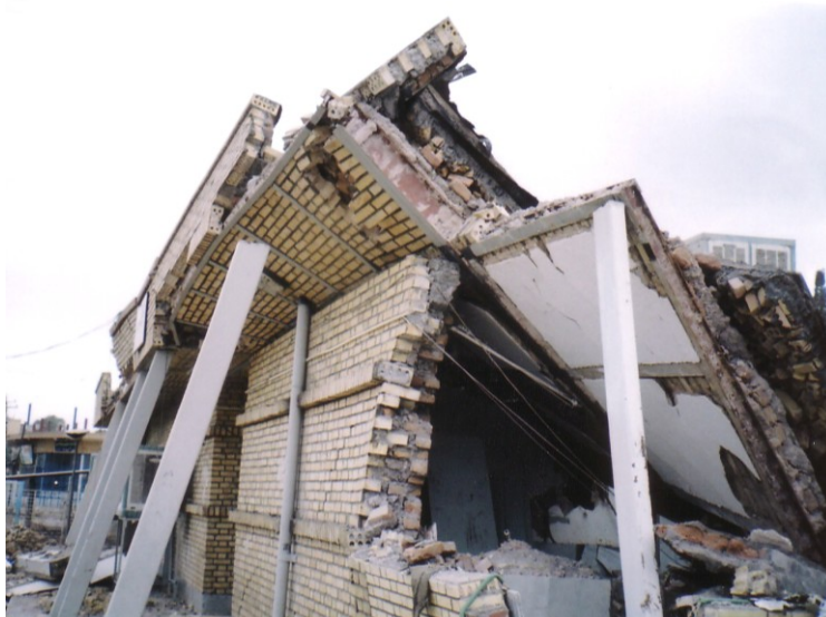
Figure 3.4. Weak columns and beams with no bracings. Photo: HFIR archive
