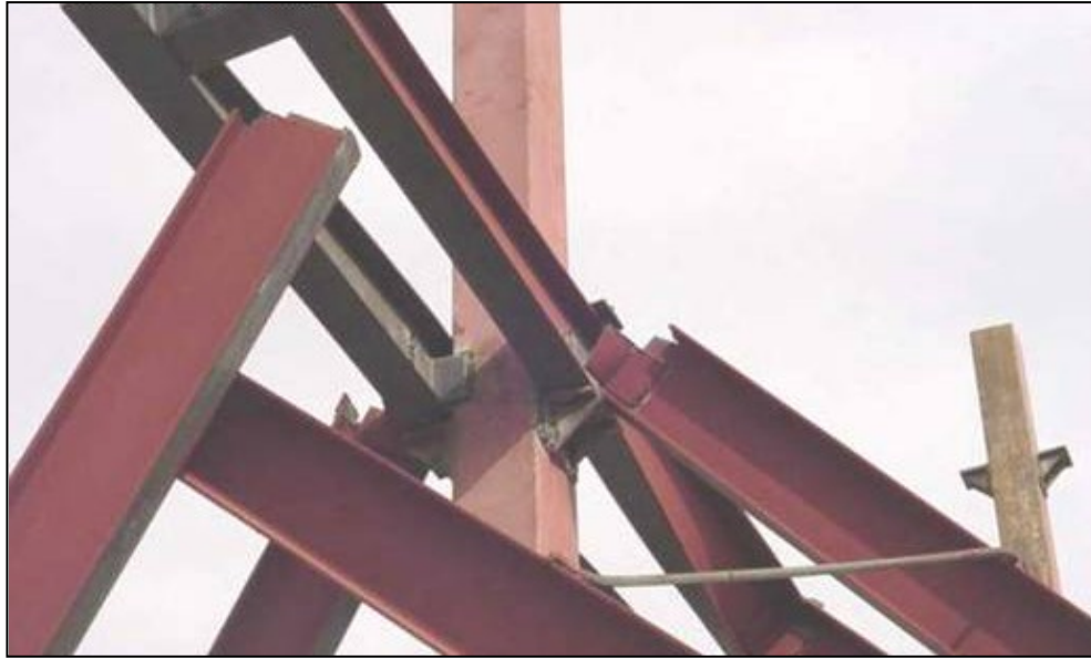
Figure 3.20. Inadequate welds at the joints was the most prevalent problem. Photo: ISEO 2004
