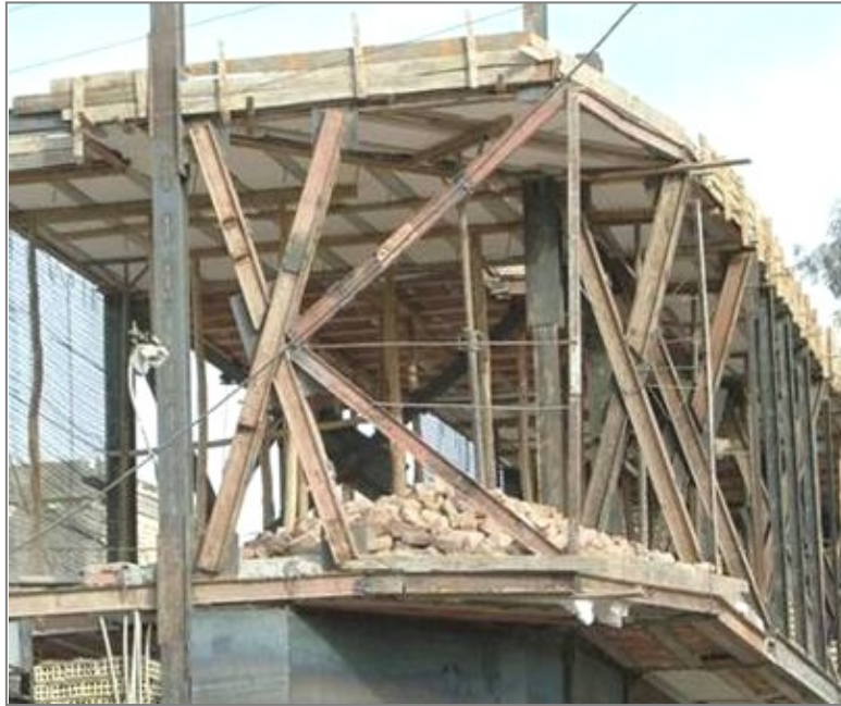
Figure 3.41. Improper use of reinforcement illustrates the presence of a blind knowledge of safe-construction.
