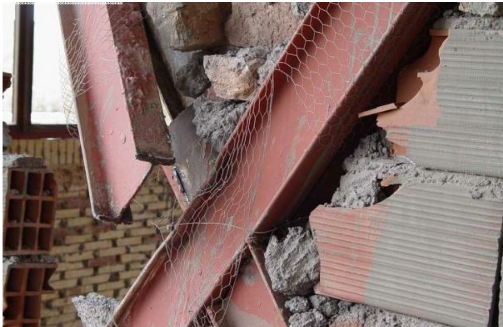
Figures 3.21. Poor quality of welding in steel construction in Bam. Photo: ISEO 2004
