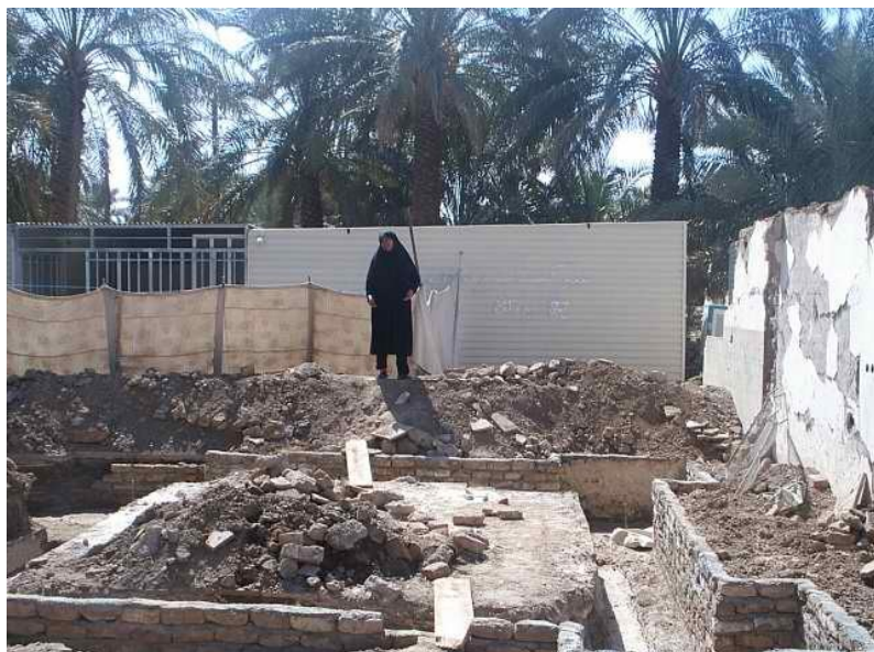
Figure C.2. After 15 months, not many houses were completely reconstructed. Photo: HFIR archive
