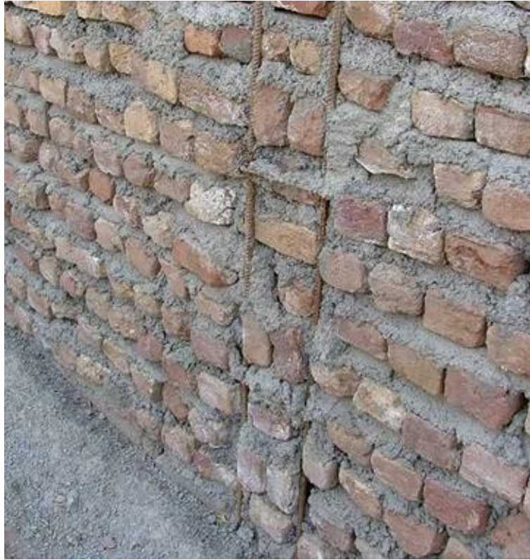
Figure 3.42. The space that was supposed to be poured with concrete to form the vertical column. Here, reinforcement is filled with bricks instead. This demonstrates an absence of proper understanding.
