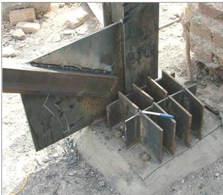
Figure 3.40. Overuse of stiffeners and gusset plates represents the citizens' fear of building collapse
