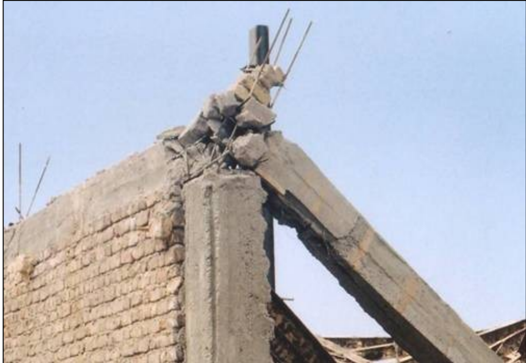
Figure 3.25. Weak junctions in a reinforced concrete-frame building. Photo: HFIR archive
