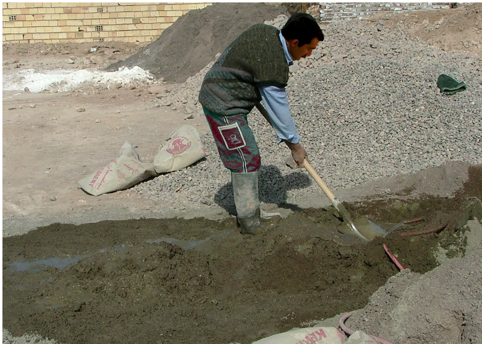
Figure 3.47. A wide variety of aggregates and fillers was available to the construction market
