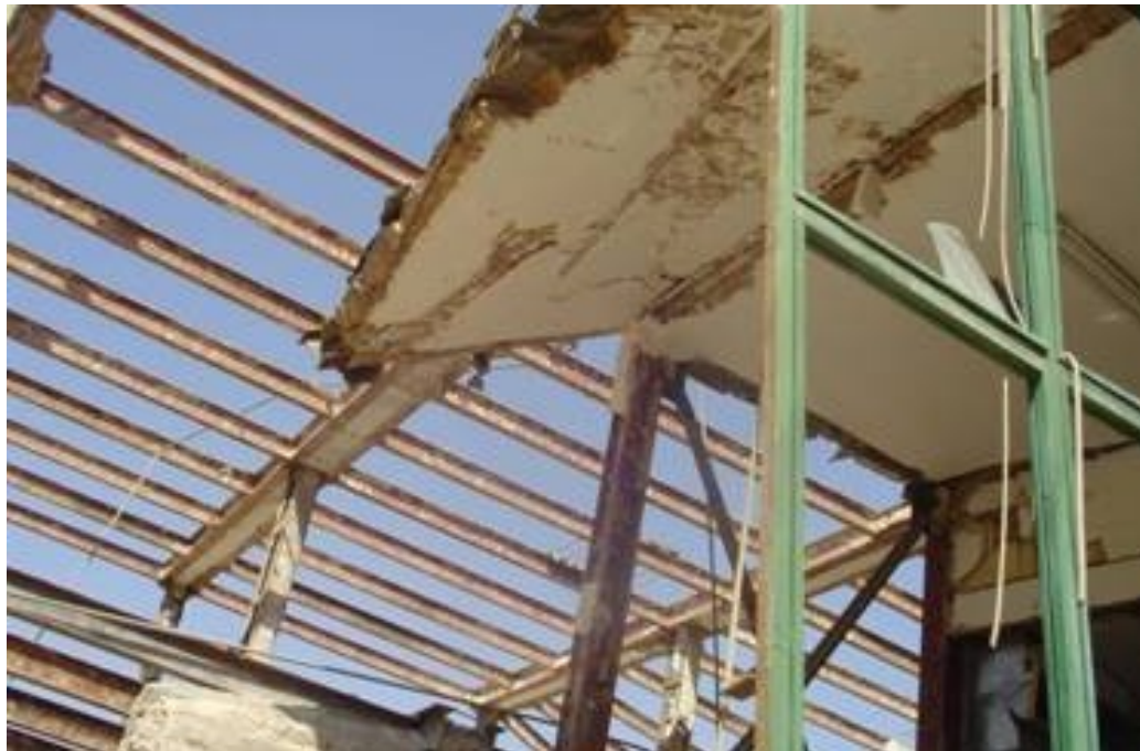
Figure 3.14. A weak bond between steel and brick resulted in the collapse of this roof. Photo: HFIR archive
