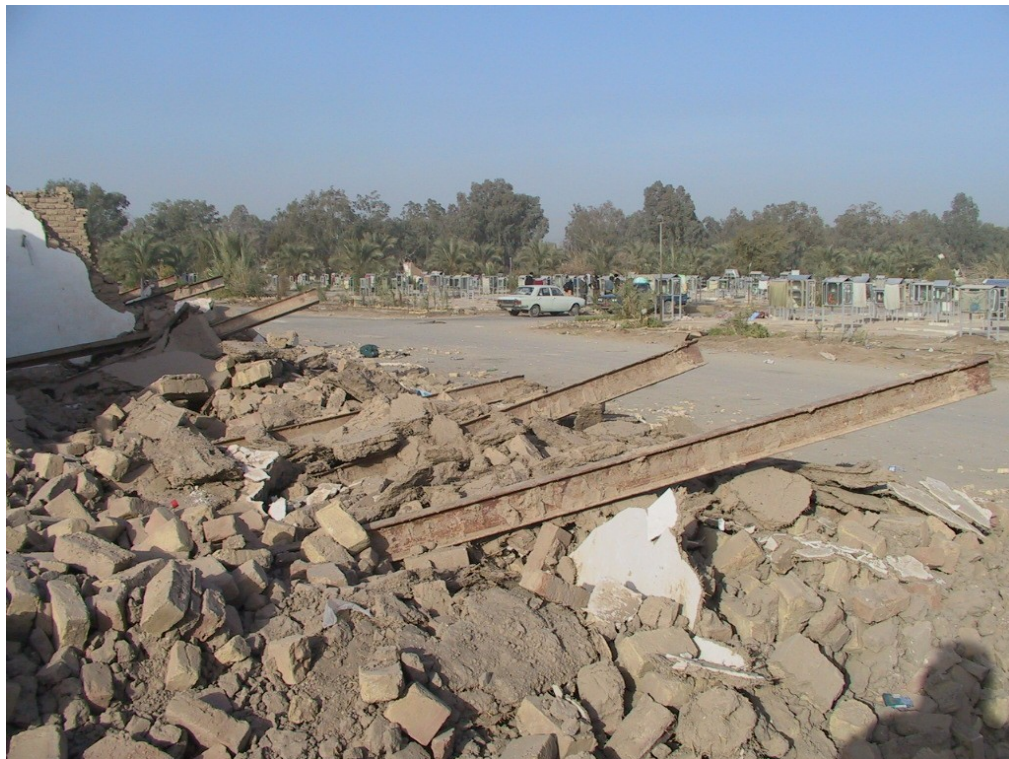
Figure 3.18. Poor bond between the bricks of the wall and the steel beams: load bearing brick walls with steel girders and a jack arch roof were destroyed completely, while the beams have remained intact. Photo: HFIR archive
