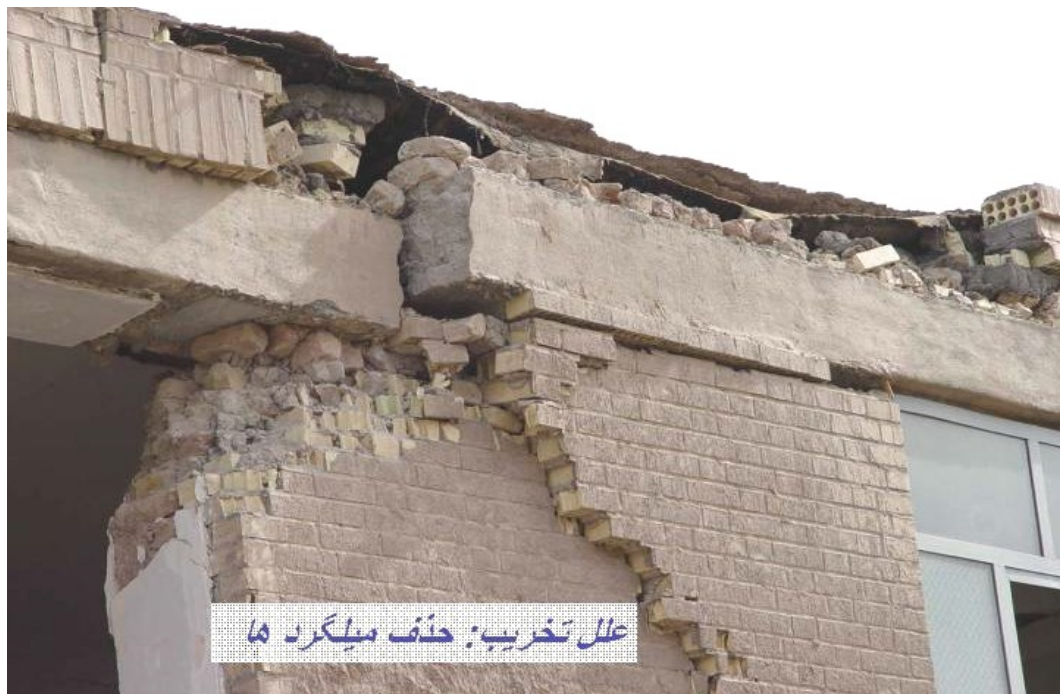
Figure 3.6. Absence of steel bars from a reinforced concrete beam. Photo: ISEO 2004
