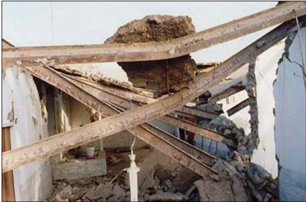
Figure 3.24 . Weak junctions in a hybrid building; steel beams resting on adobe walls. Photo: HFIR archive
