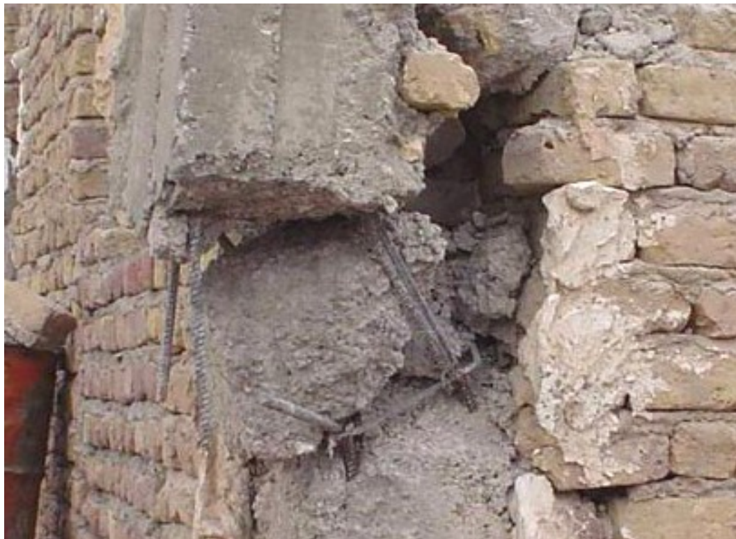
Figure 3.23. Reinforced concrete column with inadequate steel bars. Photo: HFIR archive
