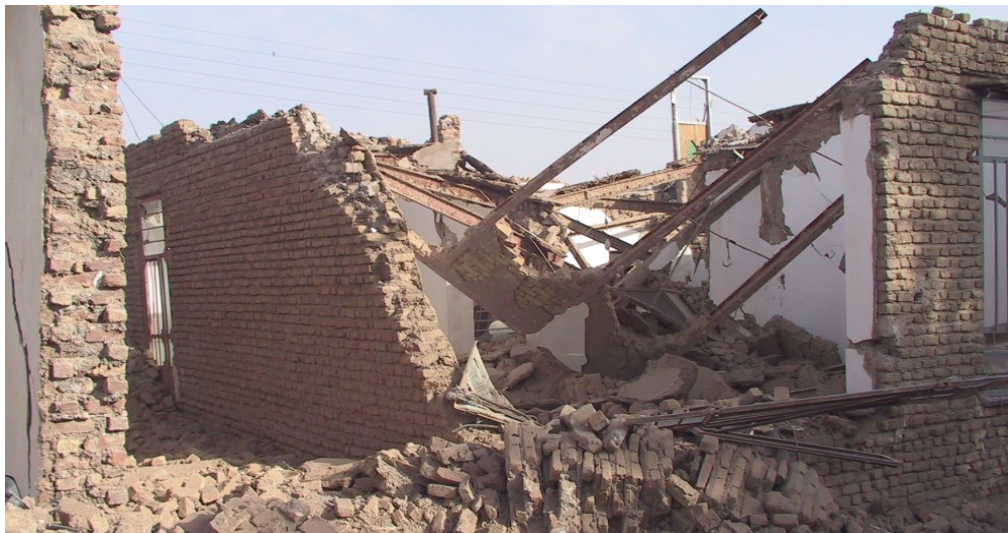
Figure 3.10. Roofing system incompatible with load bearing walls. Photo: ISEO
