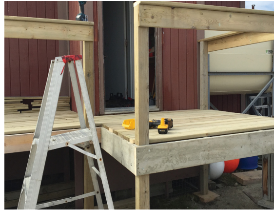
Figure 114. A skilled carpenter adds a deck to his NTR house. He moved the stair 90 degrees to park his vehicle along the front and minimize the distance to his house.
