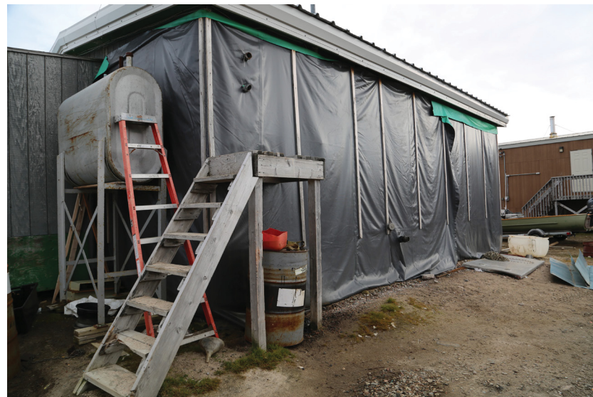
Figure 156. Northwest Territories Rental unit needing extra plastic cladding to windproof the north wall.
