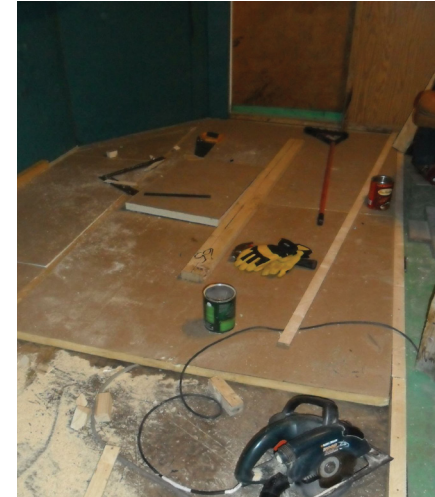
Figure 118. New insulated floor in Isaac's workshop (Tassugat, 2015). He used 2x2s, insulation, and 1/2" plywood on 2x2s.
