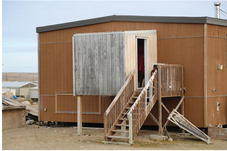
Figure 110. A 6'6" x 8' porch is added to this government house on piles, providing additional space for hanging coats and storing boots. It changes the entryway orientation from north to east and reduces snow accumulation at the front door. The stair is reused and sits on a new wood pad.
