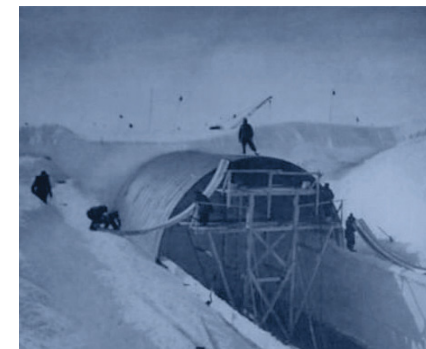
Figure 100. Quonset hut covered in snow for camouflage and added insulation, erected atop subterranean trenches for living for the US military in Greenland (Colgan et al., 2016).
