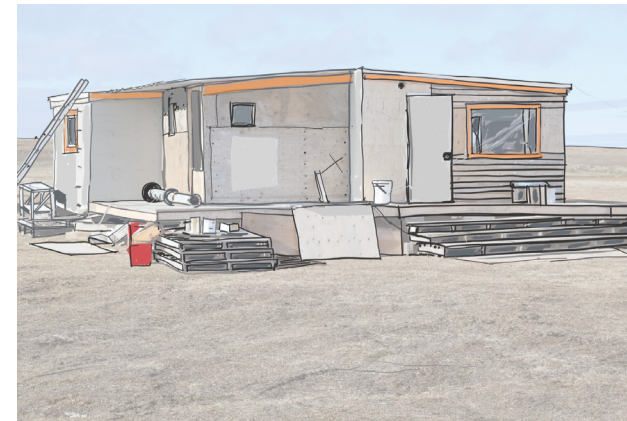
Figure 144. Respondent’s cabin during construction. Pallets are used as stairs and provisional supports. The second door is a separate porch with a honey bucket.
