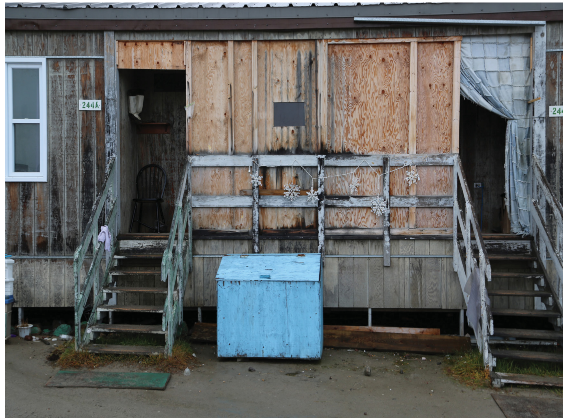
Figure 155. Recessed space between two duplexes. This was partly closed off to shelter it from snowdrifts and to provide additional cold storage.
