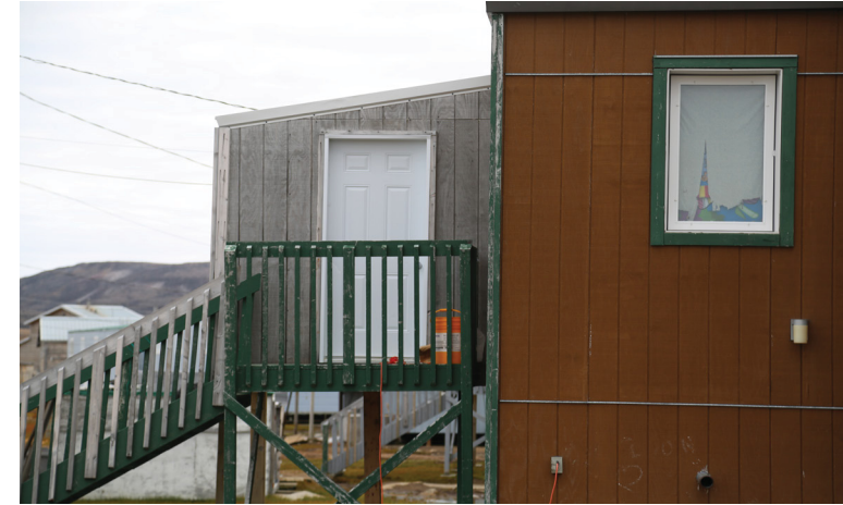
Figure 111. Added porch with its new door, shifting the entry orientation 90°. There is insufficient paint to match the original green colour for the stair handrail and trim.
