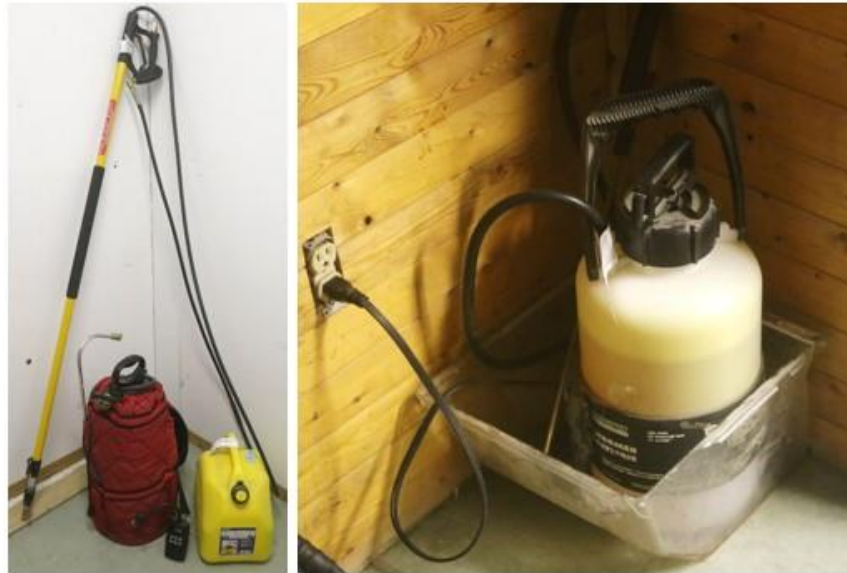
Figure 10—De-icing Equipment at FDL Airport at the time of the Crash of Flight WEW282
