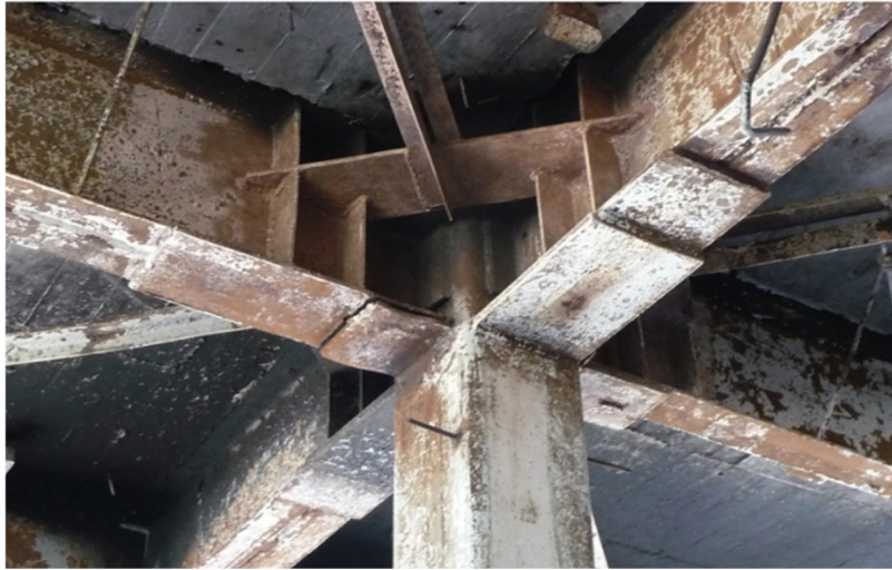
Figure 2-6 Failure of Type 2 with Wind WFP connection in Chile Earthquake 2010 (Kyriakopoulos, 2012)
