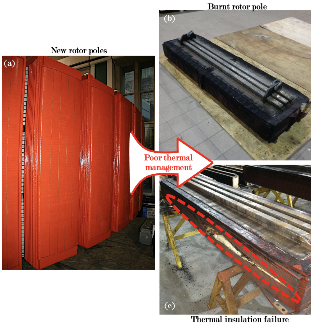
Figure 1.5: Damages to the rotor poles of a hydroelectric generator due to poor thermal management. (a) New set of rotor poles prior to their commissioning. (b) A burnt rotor pole. (c) A rotor pole with insulation oozing out due to overheating.
