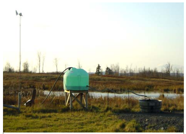
Figure 7: Stationary Solar-Powered and Wind Powered watering site
