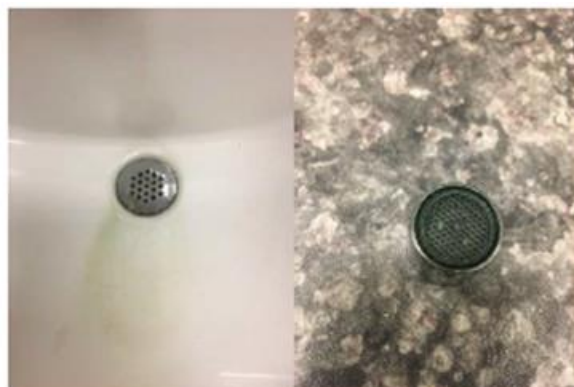
Figure 3.3 Blue stains in sinks due to leaching of copper
