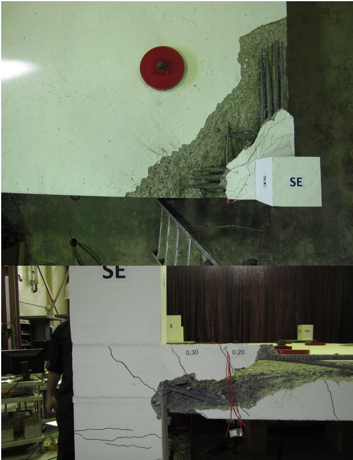
Figure 3-51: Post-punching shear condition of the corner slab-column connection SE at the end of testing
