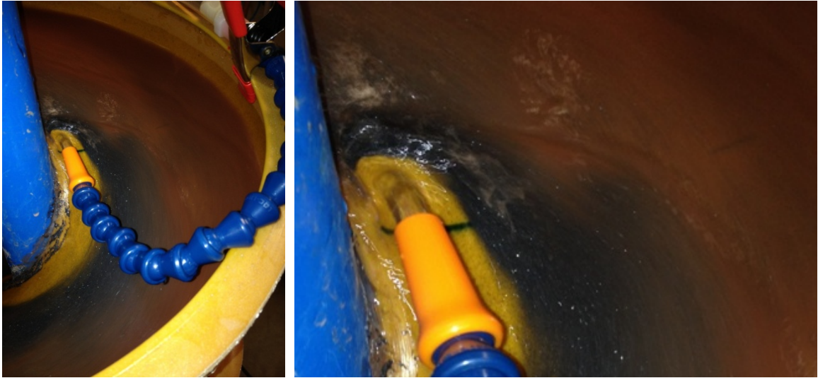
Figure 3.9 – Details of the wash water injection nozzle in the 3 rd turn during operation.
