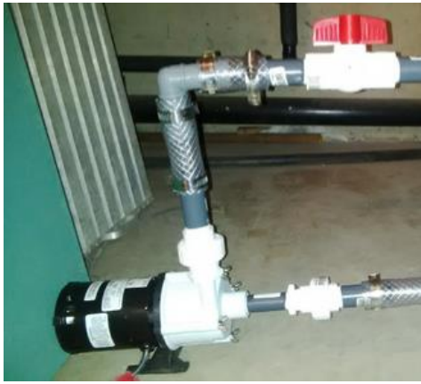
Figure 8 Picture of pump connections
