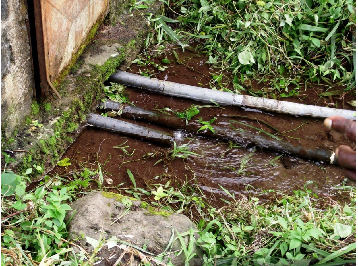
Photo 4: The outflow from tank to the network (75mm pipe) and an overflow pipe. Excess capacity is evident.
