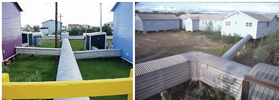
Figure 9.12 Water and sewage distribution pipes placed in surface utilidors (Town of Inuvik, 2006 on left and Photo Mondiale, 2006 on right).
