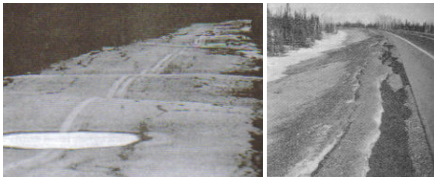
Figure 9.9 Differential settlement of a roadway (left). Longitudinal cracking of roads and airfields (right) (Esch, 1996).
