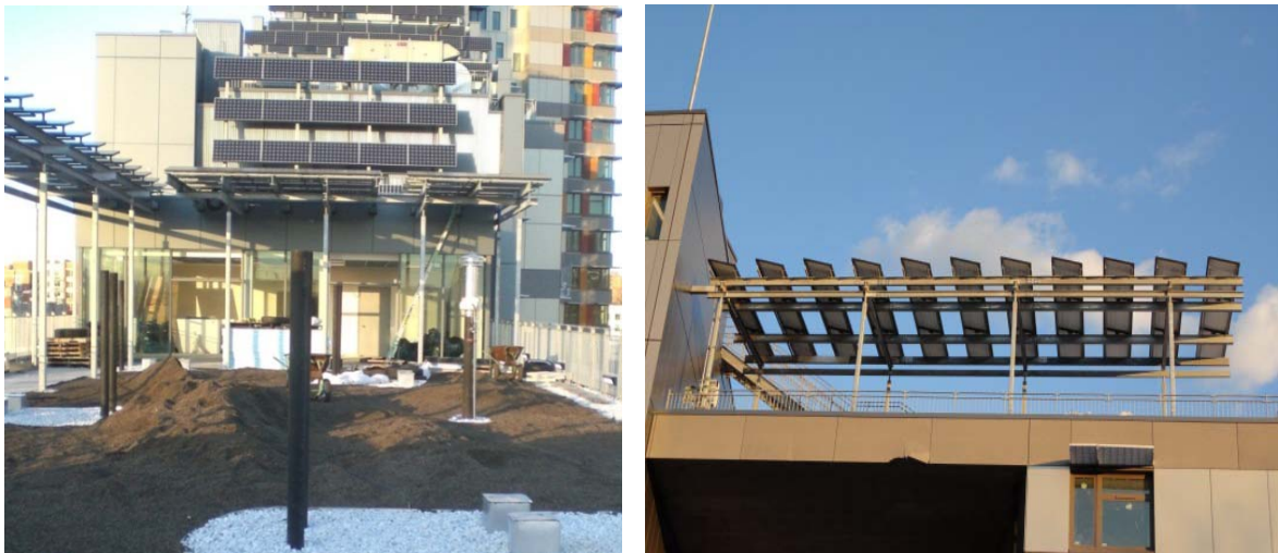
Figure 3.48: The 300 solar panels installed on the rooftop toward the south.
