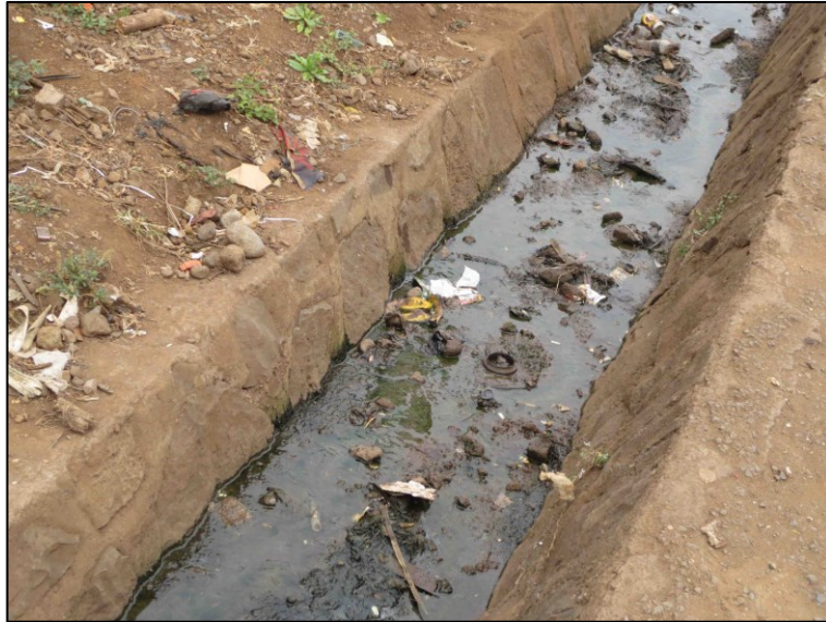
Figure 12. "Poor drainage along the major road" (Investigation Group, Buea)
