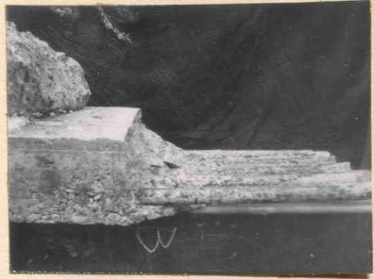
Fig. 7 Plane of failure of beam A - 1
