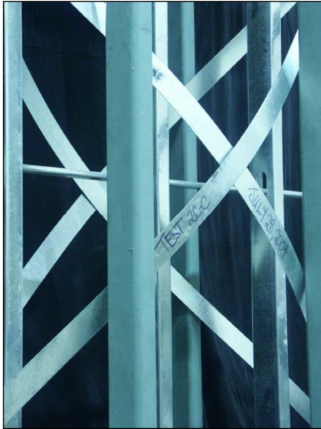
Figure 29: Magnified view of yielded 58.4 mm (2.3") strap braces after reversed cyclic testing
