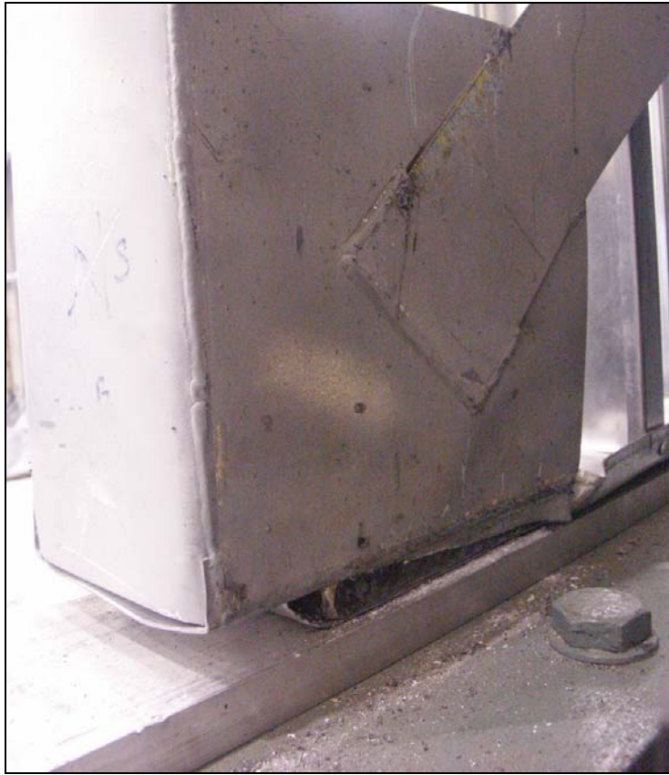
Figure 99: Punching / shear failure of bottom track : Specimen 4C-C
