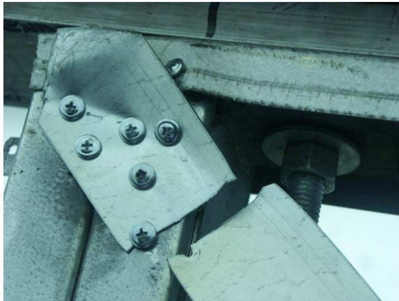
Figure 81: Net cross section failure : Specimen 1A-M
