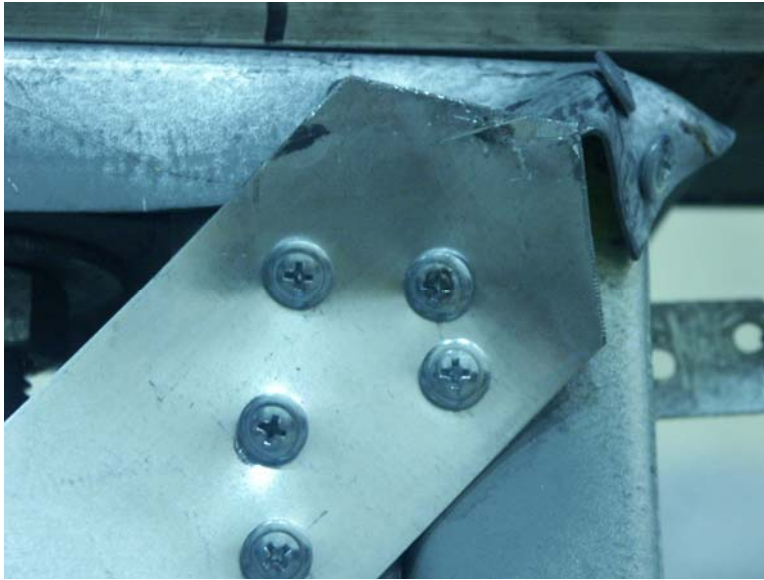
Figure 87: Chord stud to track connection failure : Specimen 2C-C
