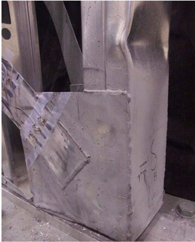
Figure 94: Local buckling of chord studs : Specimen 4A-C
