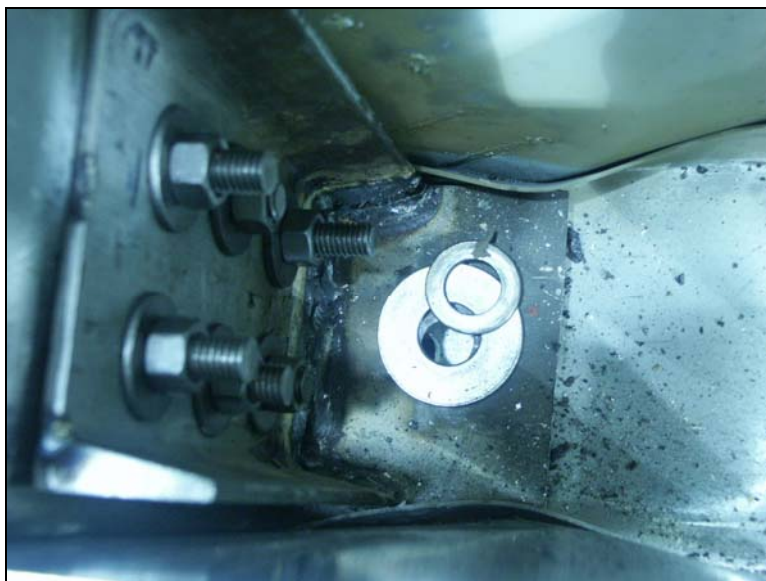
Figure 45: Anchor rod failure of specimen 5C-M
