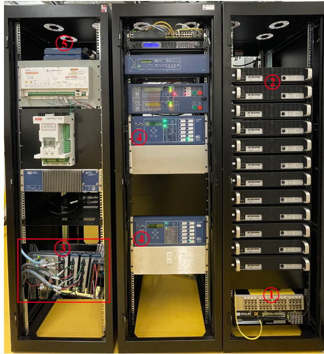
Figure 5-2: C-HIL setup, 1) RT simulator. 2) Amplifiers, 3) Controller (installed on the back of the rack), 4) Protection relays 5) Radio transceivers
